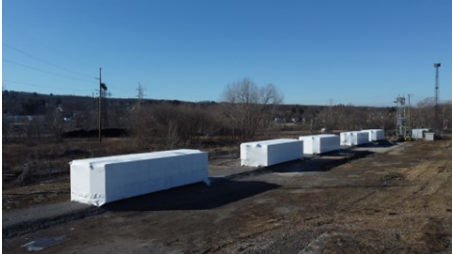
Sharon, Pennsylvania facility expansion
