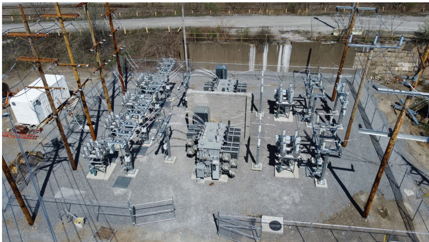
Aerial view of Midland, Pennsylvania new substation expansion
