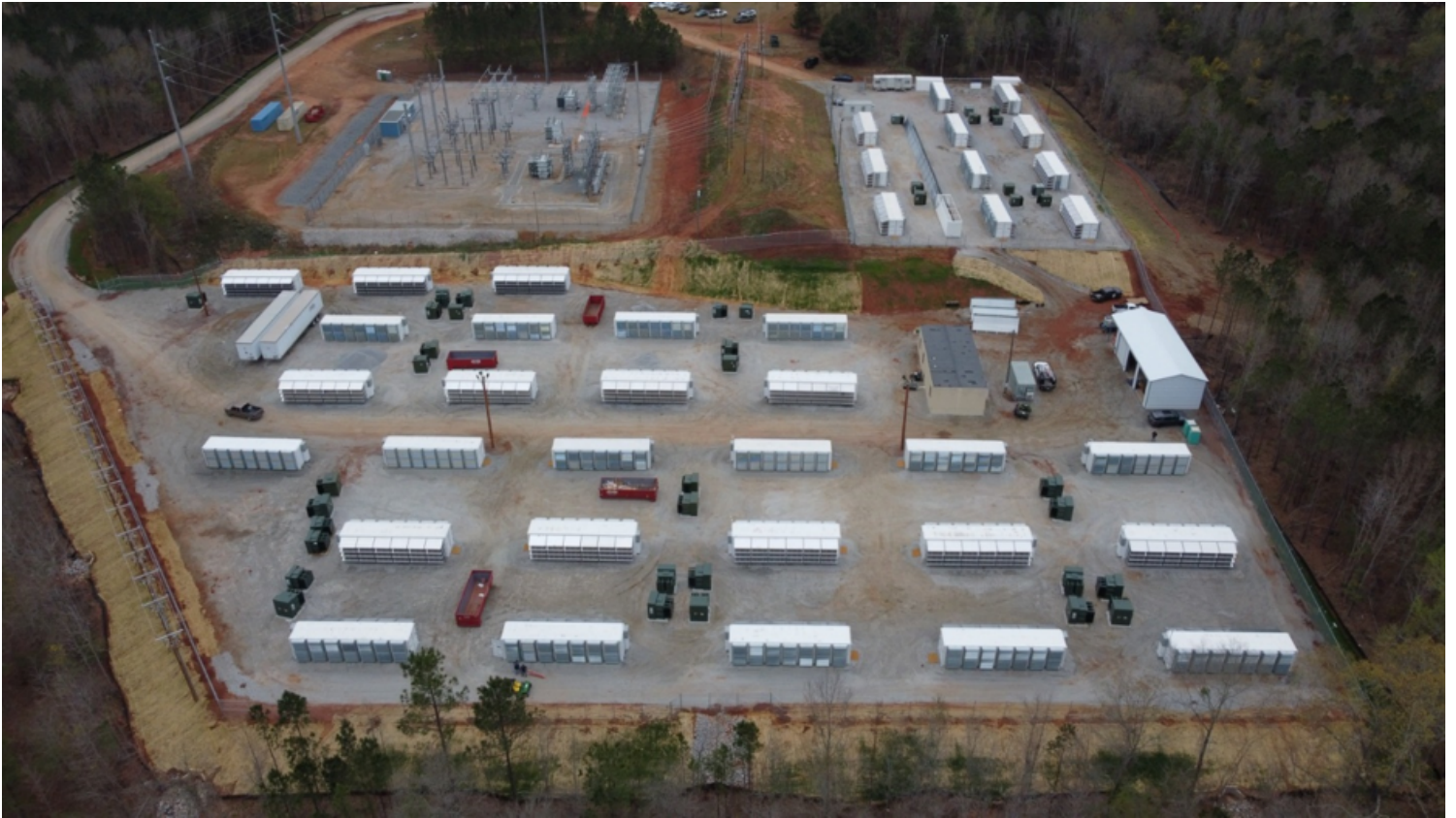
Aerial views of Sandersville, Georgia facility – 80-megawatts / 38 Modular Data Centers (April 2022)
